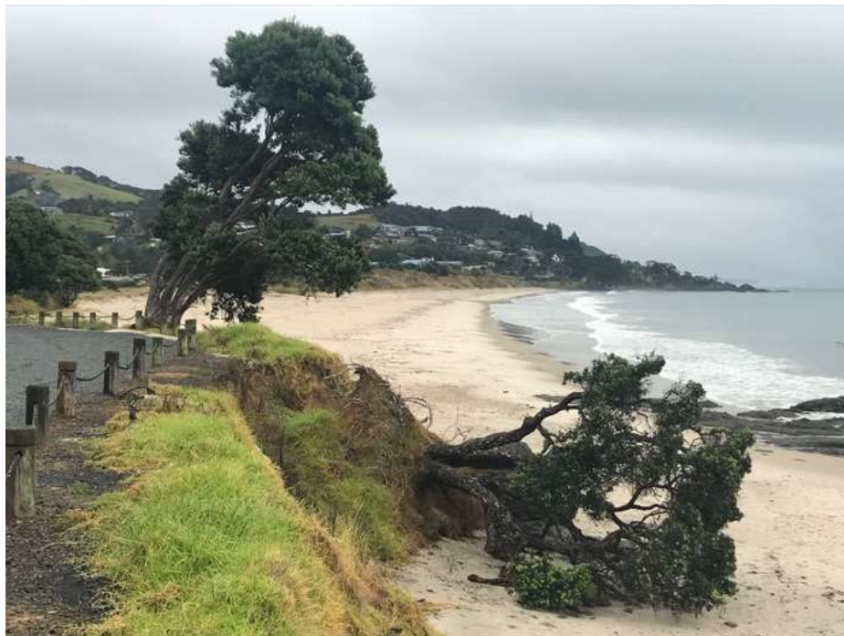
Figure 1 Recent erosion along coastal reserve frontage abutting SH 25/Kuaotunu Wharekaho Road.
